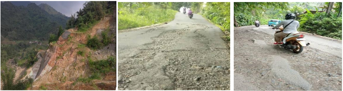
Figure 1: Road conditions in Ciasmara Village, Pamijahan District
